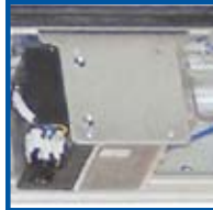
Mains supply transformer
